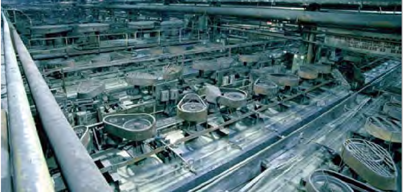
Froth flotation plant at Noril'sk. © Johnson Matthey Plc.
